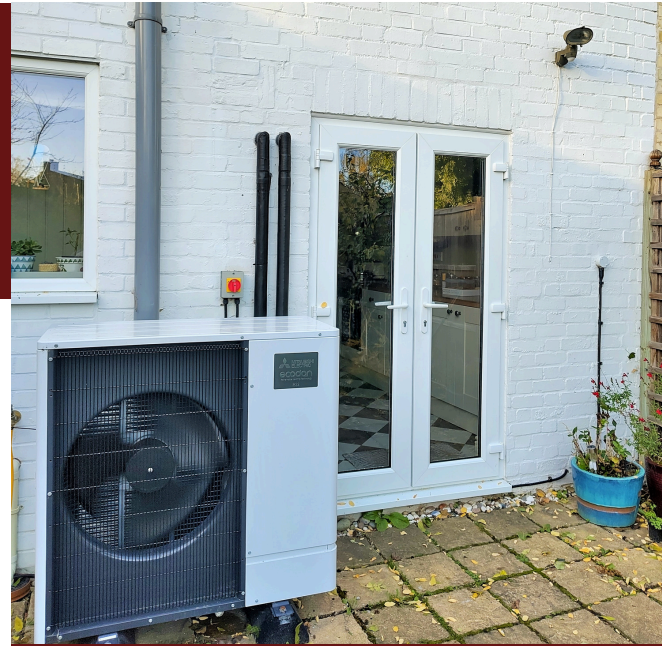
Air Source Heat Pump by back door
