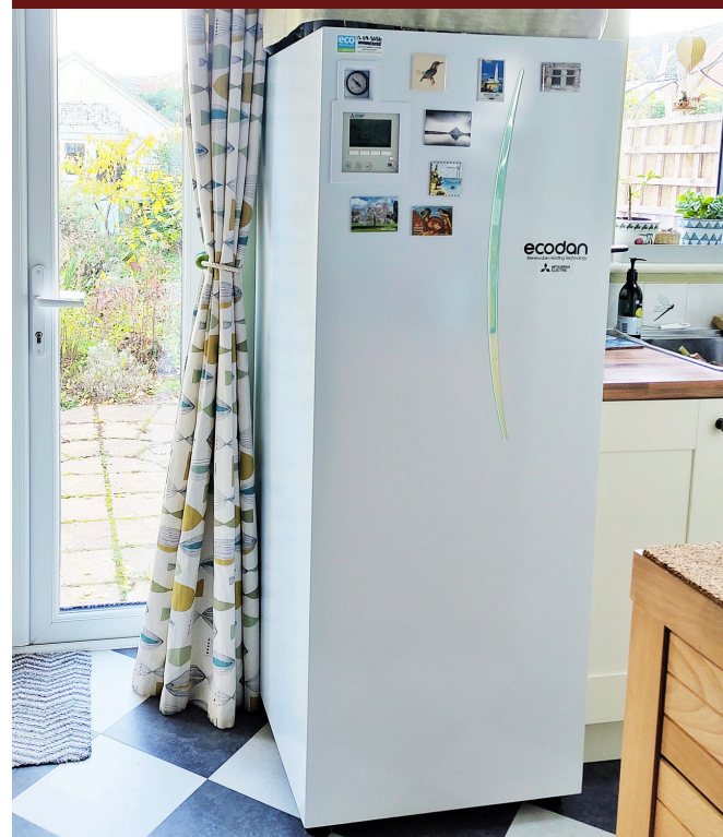
New hot water cylinder
