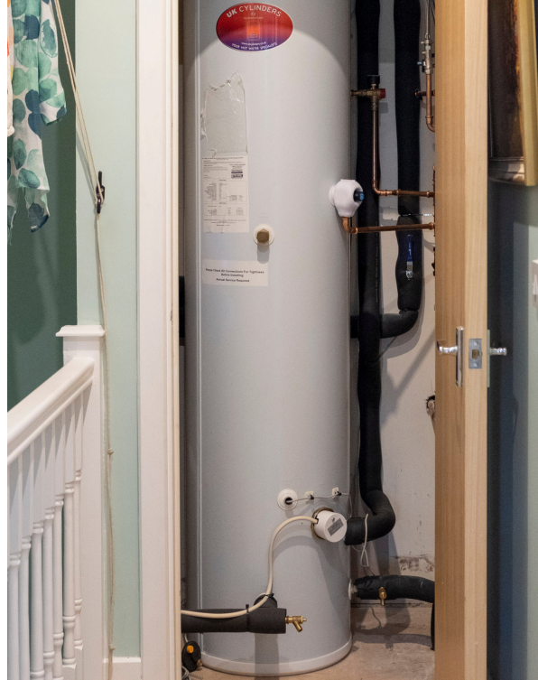
Hot Water Cylinder
