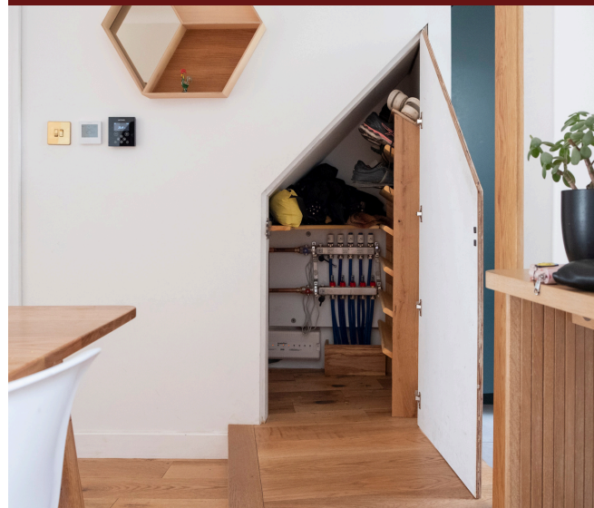
Controls in cupboard under the stairs
