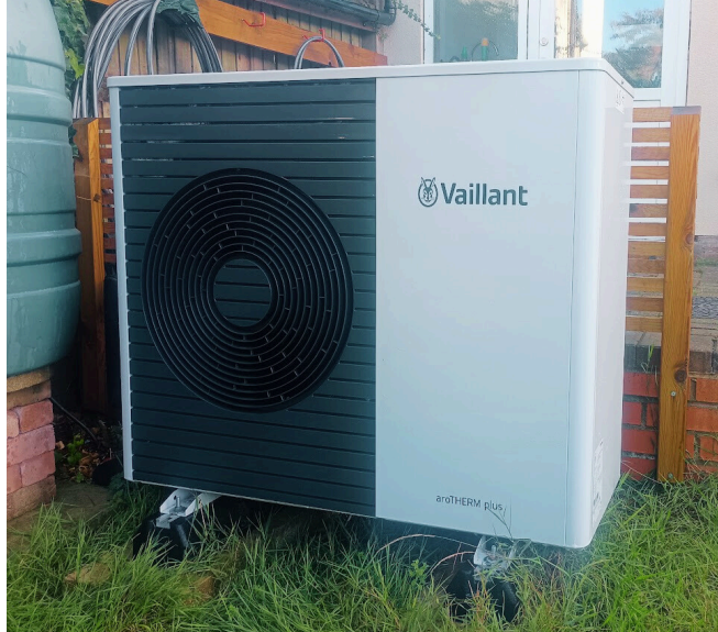
Air Source Heat Pump
