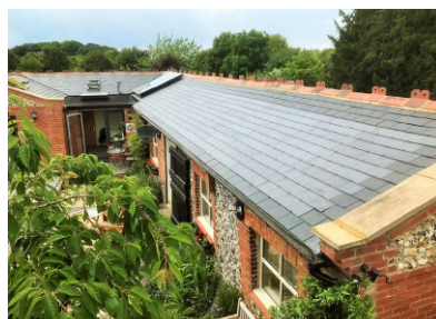
Solar PV slates
