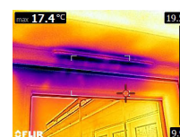
Trickle vents & door leaking heat
