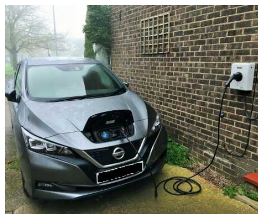
1 of 2 EV chargers
