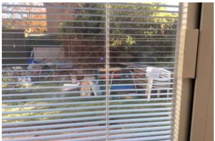
Blinds in-between the double-glazing panes
